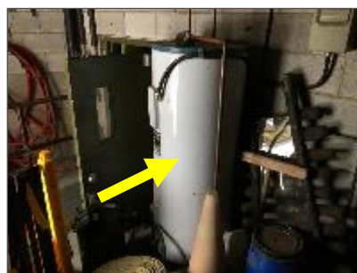
Photo 5: Hot water tank in the Storage / Mechanical / Electrical Room.
