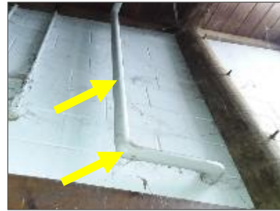
Photo 2: Pipes insulated with fibreglass and jacketed with paper and PVC in the Animal Stalls.
