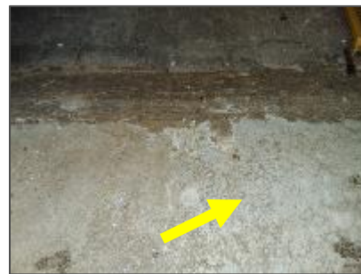
Photo 18: Grey paint on the poured concrete floor in the Storage / Mechanical / Electrical Room.
