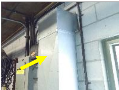
Photo 3: Uninsulated duct in the Storage / Mechanical / Electrical Room.
