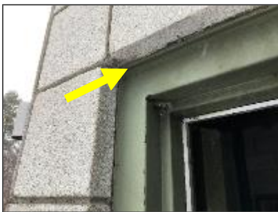
Photo 10: Non-asbestos brown caulking around the metal door frame into the Storage / Mechanical / Electrical Room.
