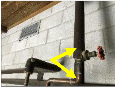
Photo 1: Pipes uninsulated and insulated with fibreglass and jacketed with paper in the Storage / Mechanical / Electrical Room.
