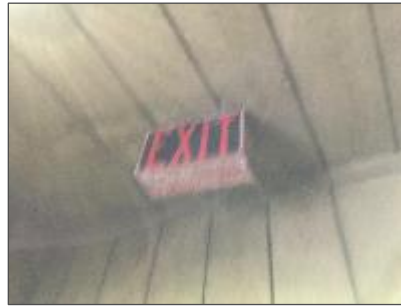
Photo 20: Emergency lighting in the Viewing Area.
