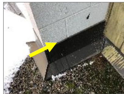
Photo 11: Non-asbestos brown caulking at the top of metal flashing on the roof.
