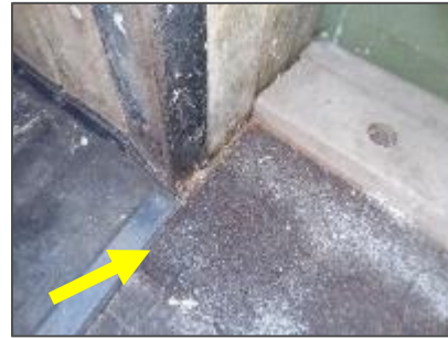
Photo 9: Non-asbestos brown caulking around the carpet floor mats in the Animal Stalls.
