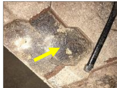
Photo 7: Non-asbestos black / dark brown caulking beneath interlocking rubber flooring in the Animal Stalls.
