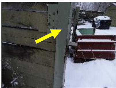
Photo 17: Green paint on the metal post at the exterior south side of the building.
