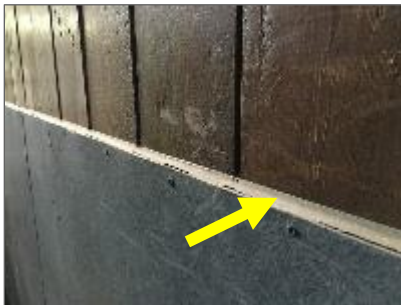
Photo 6: Non-asbestos grey caulking at top of MDF wall panels in the Animal Stalls.
