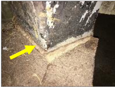
Photo 8: Non-asbestos off-white caulking at the base of metal columns in the Animal Stalls.
