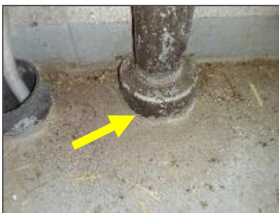
Photo 12: Non-asbestos grey caulking at conduit floor penetrations and the base of walls in the Storage / Mechanical / Electrical Room.
