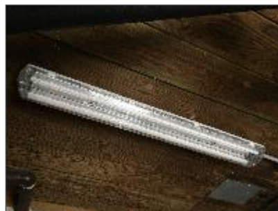
Photo 21: Fluorescent lighting in the Storage / Mechanical / Electrical Room.
