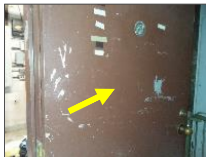
Photo 19: Brown paint on the metal exterior door frame at the entrance to the Storage / Mechanical / Electrical Room.
