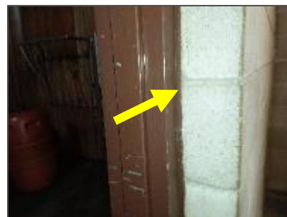
Photo 13: Non-asbestos brown caulking around the metal door frame to the Animal Stalls.
